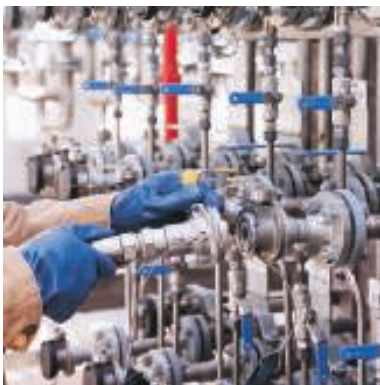
FIGURE 2. Numerous variables and components must be carefully considered when designing a loading system to ensure that leaks are kept to a minimum
