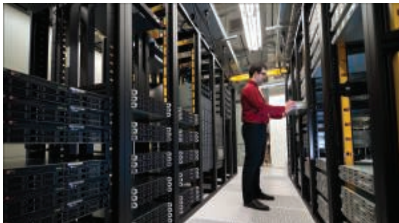
FIGURE 2. Knowing, in detail, the full extent of the facility's (and the company's) cyber assets is a critical step for developing a plan to both prevent and respond effectively to potential cybersecurity threats
